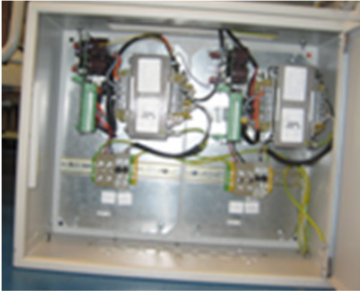
Internals of an SK box with components for 2 lights.
